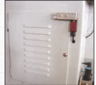
Power off device (door unclose)
